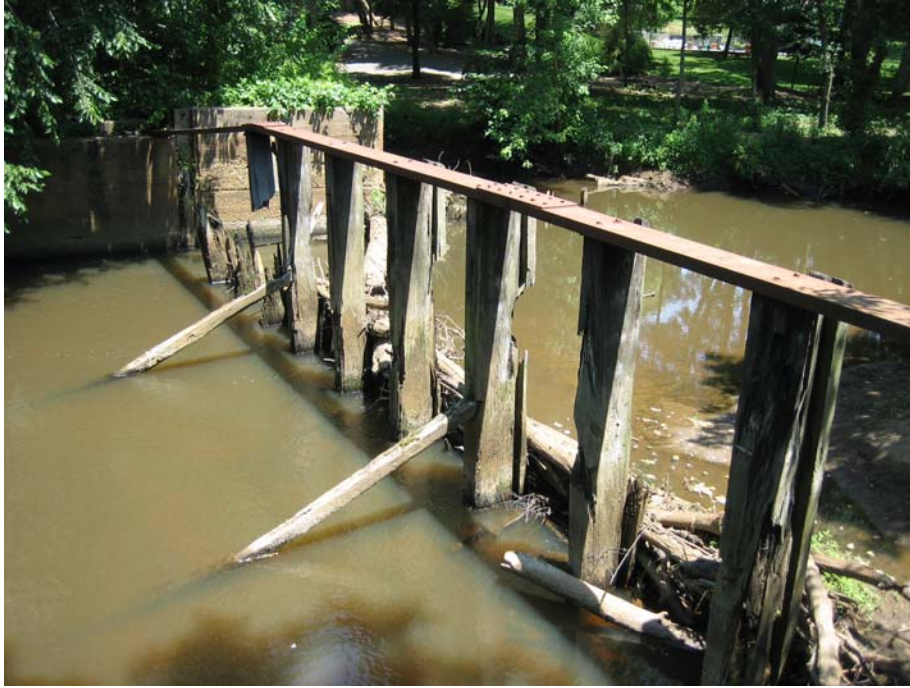
Photo 77: The downstream side of the ice house dam, viewed from the Township-owned parcel, facing slightly upstream (east).
